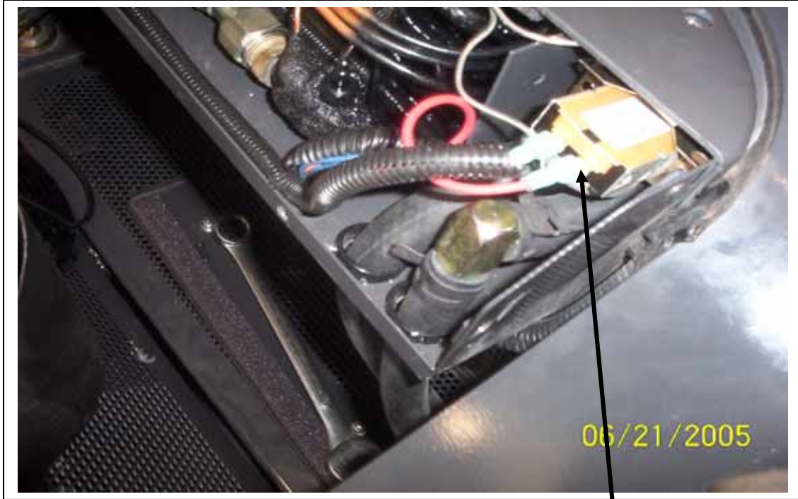
Thermostat located at the evaporator.
